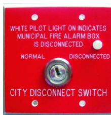
City Disconnect Switch
